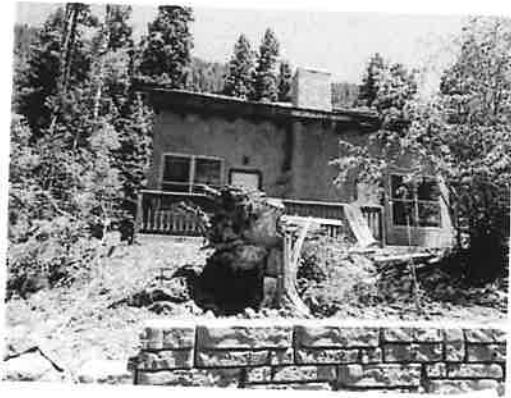
Storm damage to duplex
