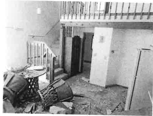
West unit 8 storm damage
