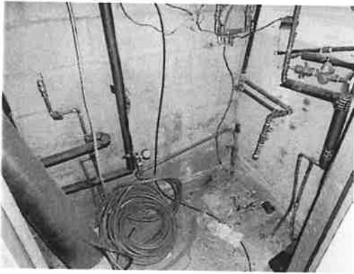
Former lodge/office boiler and capped plumbing
