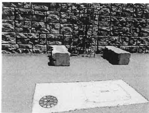
New natural gas service and well valve
