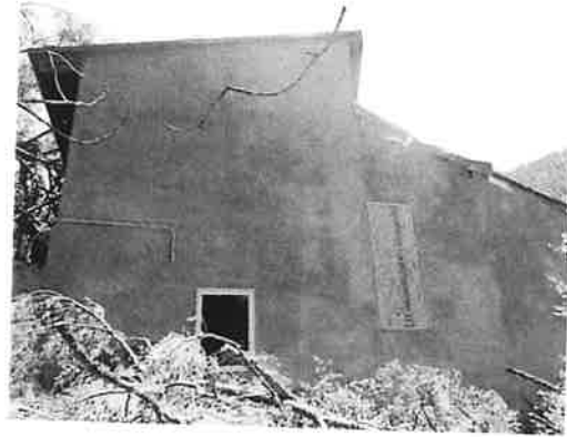
West wall of duplex and storm damage
