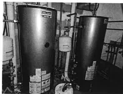
New gas boiler tanks in 8-plex
