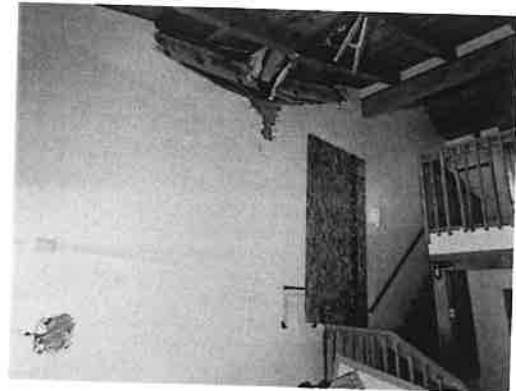
Roof damage to duplex
