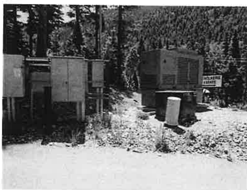
New electrical service and back-up generator (not connected)
