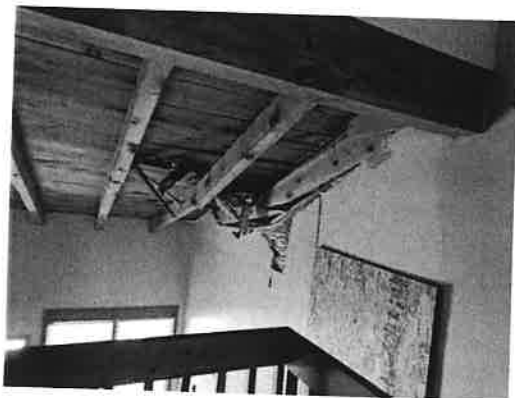
Roof damage to duplex
